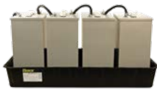
Battery tray with four L16/GC2 batteries 120220
